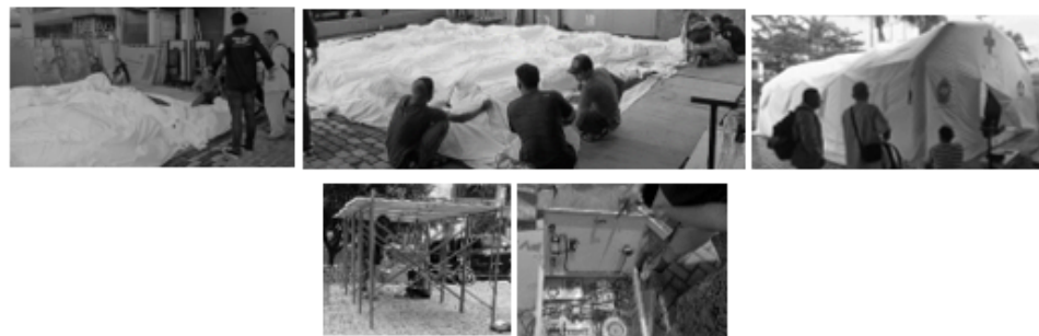
Figure 2: Construction of an inflatable tent with photovoltaic power plant.
